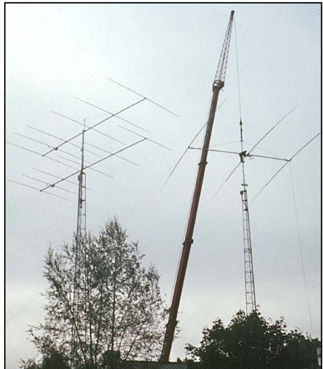
Fig 13-16 — The ON4UN 40-meter Yagi is lowered on top of the rotating mast at a height of 30 meters using a 48-meter hydraulic crane.
