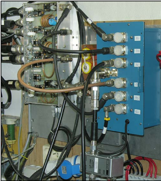
Fig 15-8 — On the left are the selector/combiner unit for 10 through 40 meters. The feed lines ( \frac{7}{8} -inch) from the single-band antennas and the 10-15-20-meter tribander (C31XR) arrive on the left. From top to bottom: 40, 20, 10 and 15-meter L-networks. There are 15 relays in the box. On the right are four band outputs for 10 through 40 meters, which go to a home-built switch box with both N connectors and \frac{7}{16} inch connectors.
