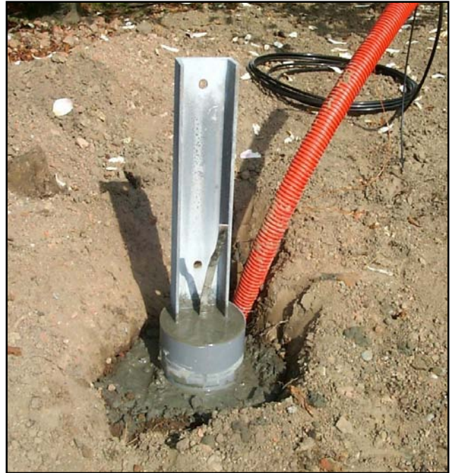
Fig 7-17 — Concrete base for the self-supporting elements used by the author. The concrete base goes down about 0.75 meter.
