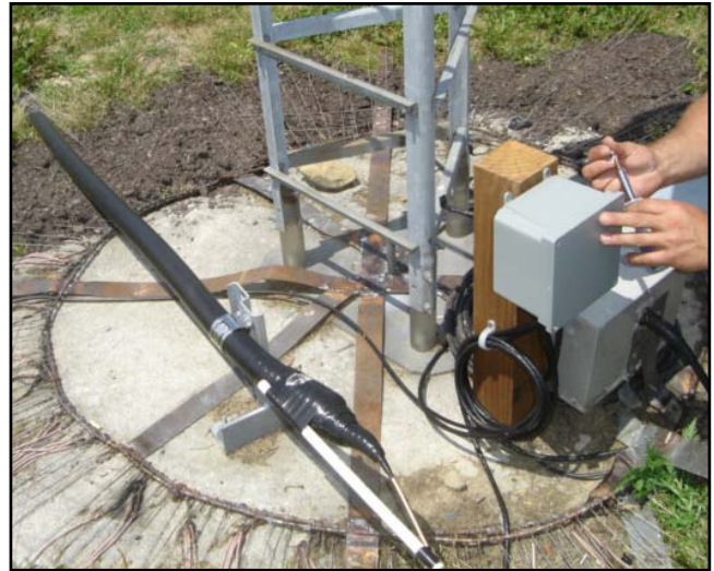
Fig 13-62 — Base insulated feed point of the 3-element K3LR vertical Yagi for 160 meters. The aluminum box contains an L network to transform the array impedance (about 25 \Omega ) to the 50 \Omega Hardline impedance (1 5/8 inch feed line!). The plastic box distributes the relay control wiring to the parasitic element relays. The coaxial cable coil to the right is a \lambda/4 shorted-stub that serves as a static drain and also provides attenuation of the 80-meter harmonic. This is very important at a multi-operator contest station! Note the 120 radials connected to the annular ring.
