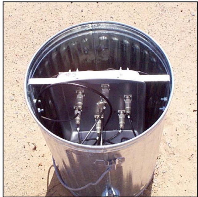
Fig 7-53 — A 10-gallon garbage can is used to house K8BHZ's phasing/switching circuitry, as well as the extra phasing-line coax (coiled up at the bottom of the can). The can is grounded using two 2.4 meter long ground rods.
