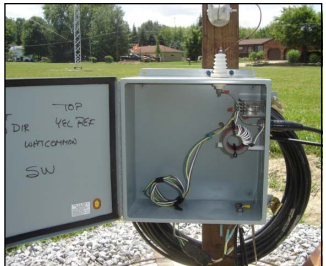
Fig 13-63 — A metal box contains the T-200-2 loading coil for the reflector mode and two small relays to switch the coil in and out of the circuit at each of the four parasitic element bases. The base of each parasitic element is also equipped with a \lambda/4 coaxial stub and complemented with no less than 120 \lambda/4 radials.
