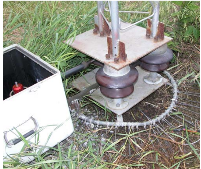
Fig 9-26 — W8LRL uses a copper tube (about 10 mm in diameter) bent in a circle, to which he solders all his radials. For a permanent installation this is probably the best way to go, provided you use silver solder or protect your connections made with regular electronics solder with liquid rubber.
