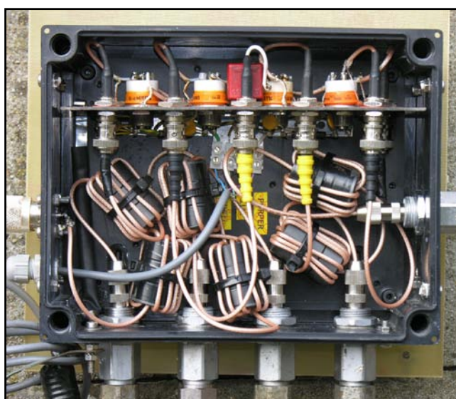
Fig 7-101 — Coaxial feed line distribution box for Beverage system. A 7/8-inch main feed line (180 meters from the shack) is fanned out to five smaller (1/2 inch) feed lines. Notice the small vacuum relays and six common-mode chokes used.
