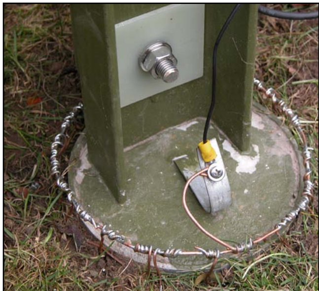
Fig 7-45 — Base of a vertical. All copper radials are soldered to a copper ring, and connected to the strap going to the 1.5-meter long ground rod.
