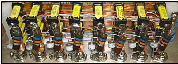
Fig 7-56 — Receiving antenna switching matrix (8 x 4 lines = 32 SPST relays) using low-cost hermetic reed relays. Note also the 90-V gas discharge tubes and the static drain resistors (56 kΩ). This relay matrix is made by Charlie, NØTT and used at his Nine Circle array (see Section 1.33)
