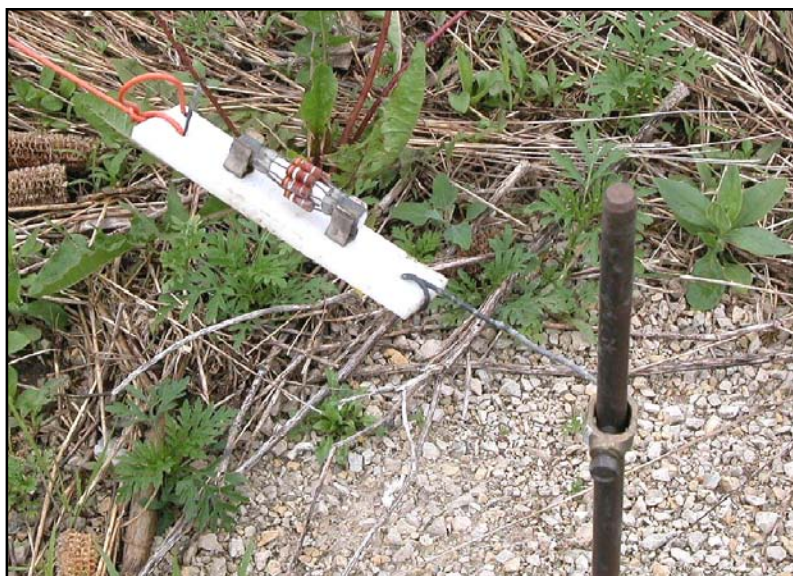
Fig 7-89 — K9DX uses a fuse clip and parallel carbon resistors soldered across a blown fuse. This makes replacement, in case of lightning strike destruction, very easy.
