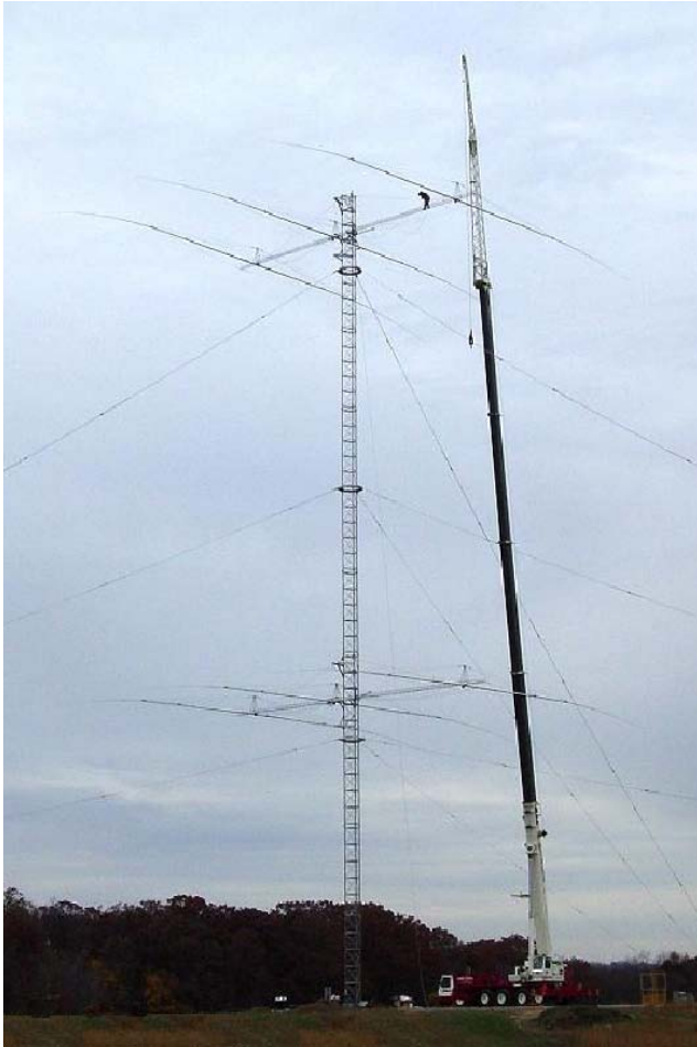
Fig 13-32 — NO8D has a stack of two 3-element full-size 80-meter Yagis that use a lattice structure as boom. This approach makes it possible to make a strong boom that weighs much less than a boom made of large diameter heavy wall aluminum tubing.
