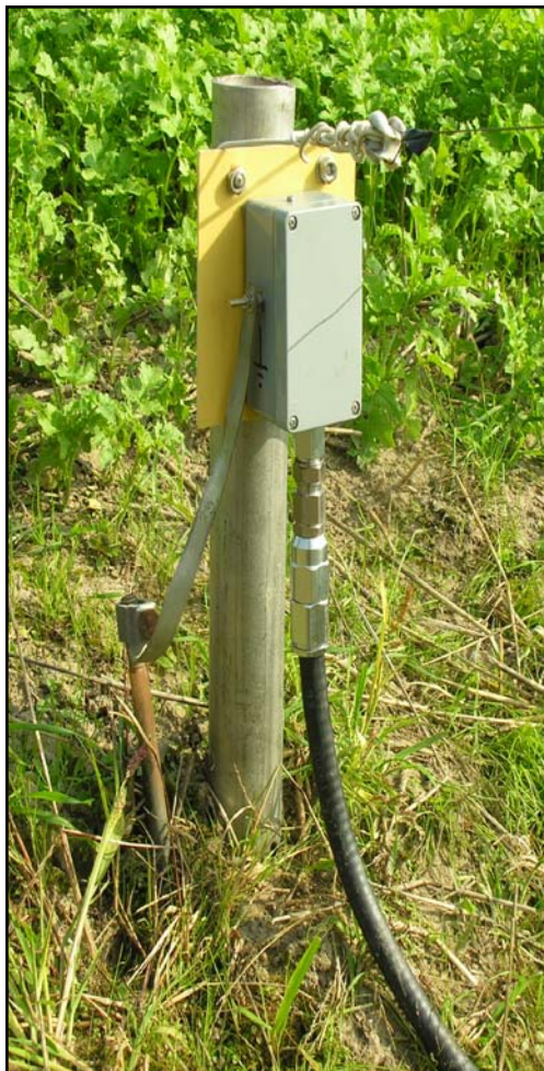
Fig 7-105 — Sloping down-lead termination for one of the Beverages at ON4UN. A stainless steel pipe supports the feed box that contains the binocular transformer and the common-mode choke. Note the 1/2 inch 75-Ω feed line and the professional grade connectors used. To the left we see the top of a 15 mm diameter copper rod driven into the ground, to which a tinned copper strap is connected. This provides the ground connection to the transformer.
