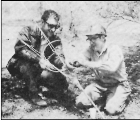
Fig 23—A length of guy cable is used to assure that the turnbuckles remain in place after they are tightened. This procedure is an absolute requirement in guyed tower systems. (Photo by K1WA)
