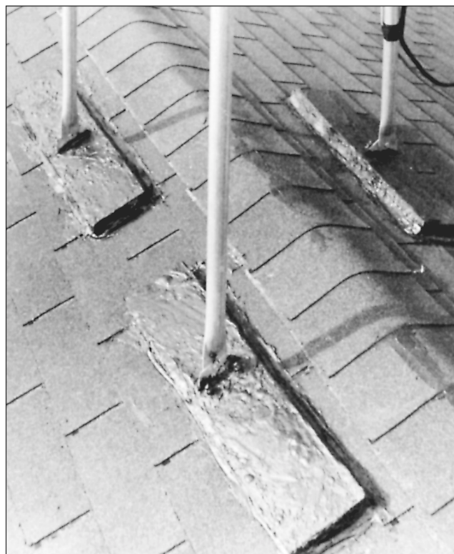
Fig 44 —Three lengths of 2 × 6 wood mounted on the outside of the roof and reinforced under the roof by three identical lengths provide a durable means for anchoring the tripod. A thick coat of roofing tar guards against weathering and leaks.
