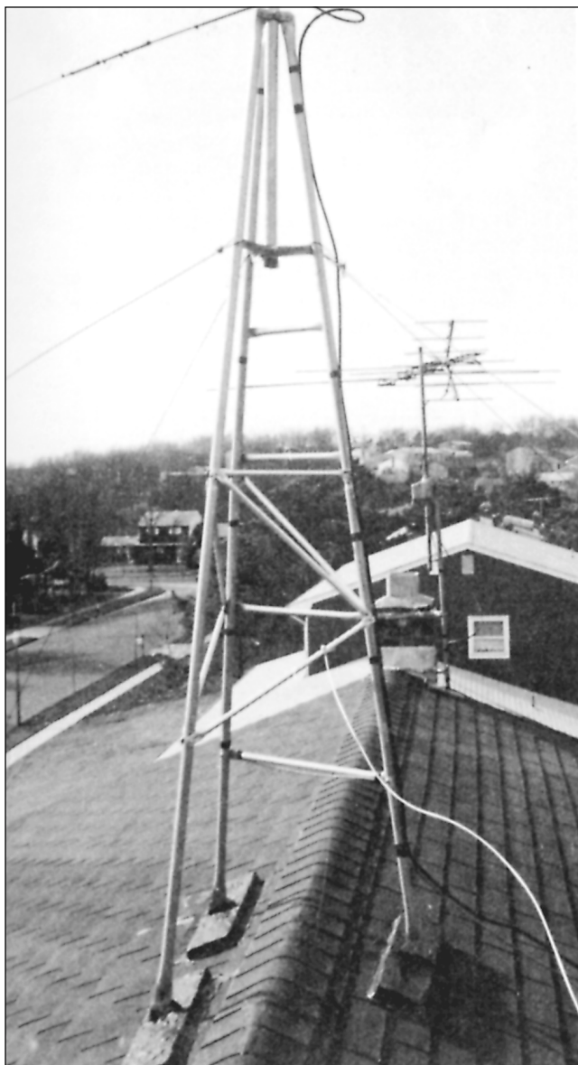
Fig 42 —This tripod tower supports a rotary beam antenna. In addition to saving yard space, a roof-mounted tower can be more economical than a ground-mounted tower. A ground lead fastened to the lower part of the frame is for lightning protection. The rotator control cable and the coaxial line are dressed along two of the legs. ( Photo courtesy of Jane Wolfert )
